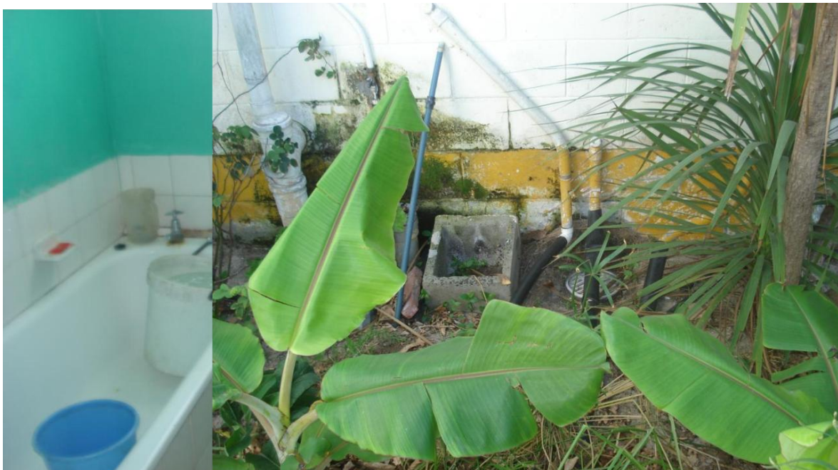
Figure 2: Grey water recycling system with papyrus plants for water filtration with pre-existing banana trees in the foreground
